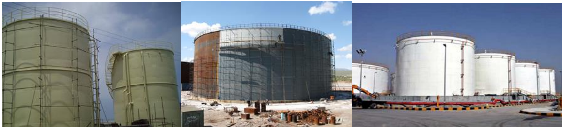
Figure (1) Use of steel reservoirs in oilfield plants and refineries
